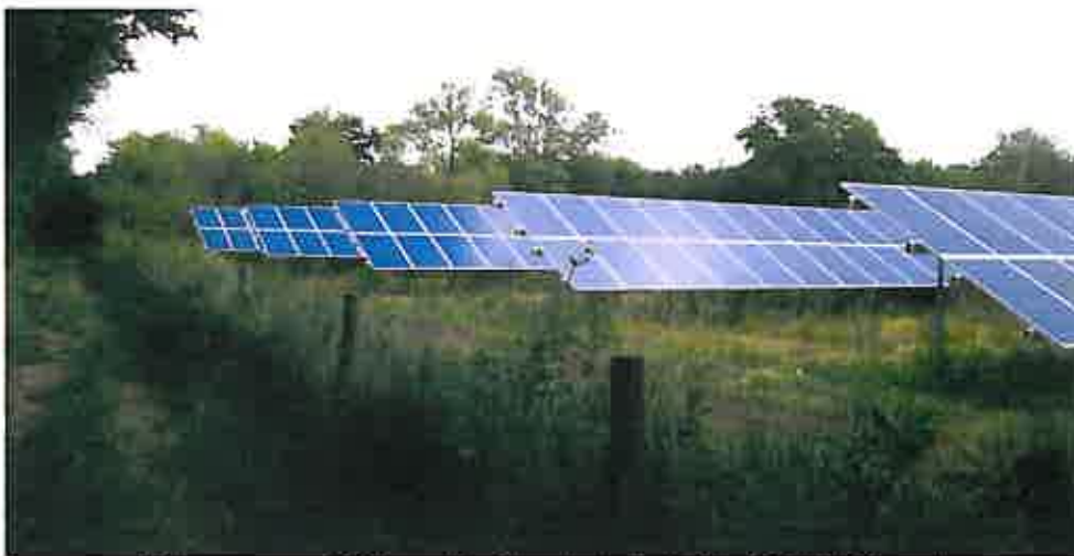
Solar arrays. © Olwen Maidment, Teignbridge District Council
